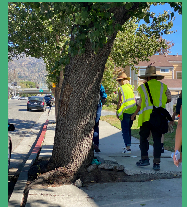
Figure 5. Insufficient tree well size
