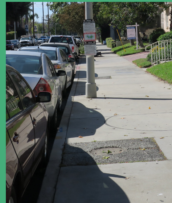
Figure 4. Tree well obstruction
