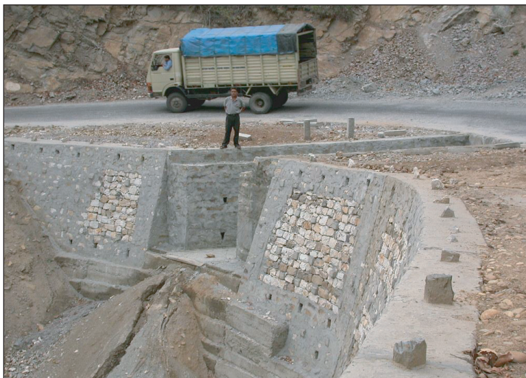
Figure 7. Construction of big culvert and check dam for proper drainage throughout the length of the road passing along the Upper Ganges.
