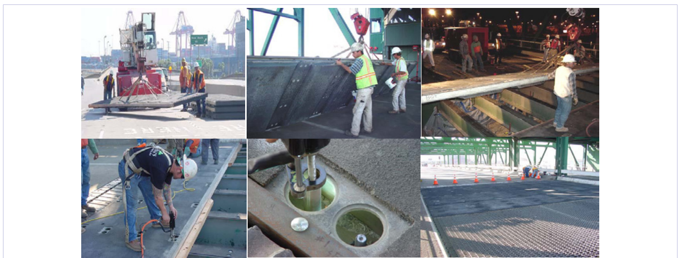
Figure 36: Field installation of the hybrid composite bridge deck at the Schuyler Heim bridge site, Long Beach, California, USA.
