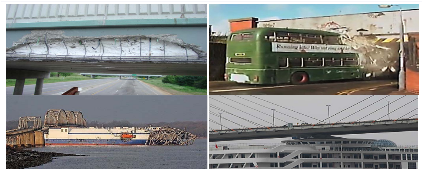
Figure 13: Impact damages in the concrete bridge girders by over-height trucks and buses.
