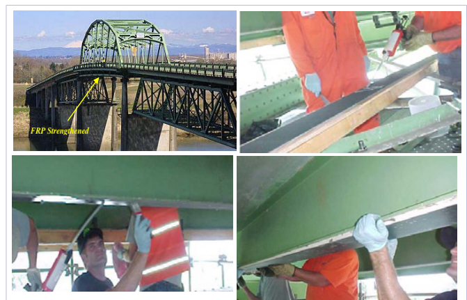
Figure 22: Field application of the h-lam system for the sauvie island bridge, Portland, Oregon, USA.
