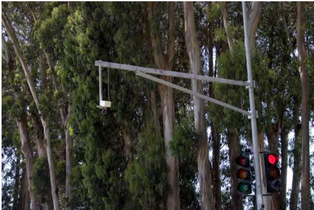
Figure 23. Road Traffic Microwave Sensor by Electronic Integrated Systems
