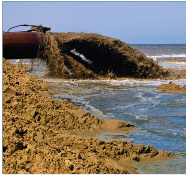
Figure 4.4 Sewage discharge into a receiving body. In older cities, wet weather events can overload combined sewage systems causing untreated sewage discharge into local waterways.
