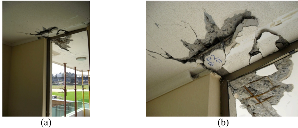
Figure 3.18 Second story damage in axis C, between 13 and 14: (a) view 1; (b) view 2.
