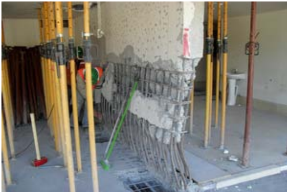
Figure 1.1 Buckled wall in first story of Alto Huerto building (DICTUC report #906575/10-056-EE-01-R0, 2010).
