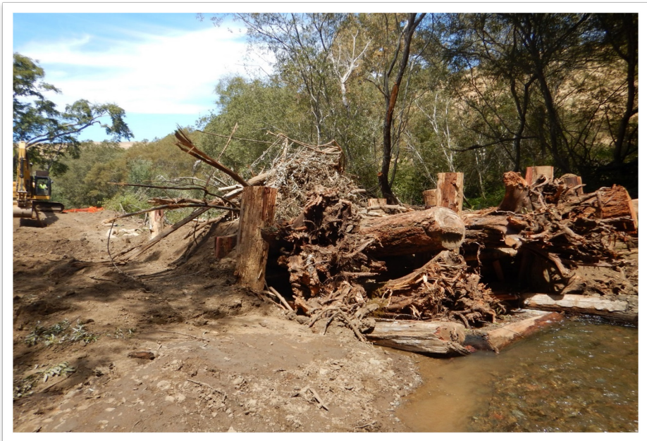
Figure 25. Large wood project using a piling for stabilization. Photo credit: Greg Andrew, Marin Municipal Water District.
