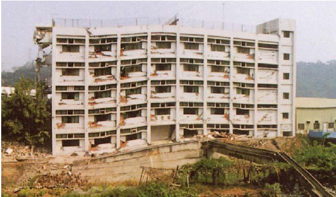
Figure 2-9. A building heavily damaged as a result of surface fault rupture during the 1999 Chi-Chi event (GEER 1999).
