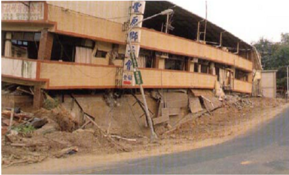
Figure 2-11. A building that partially collapsed likely as a result of surface fault rupture during the 1999 Chi-Chi event (GEER 1999).
