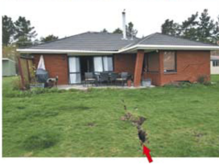
Figure 2-18. Building damage as a result of surface fault rupture from the 2010 Darfield, New Zealand Earthquake (Van Dissen et al. 2011).
