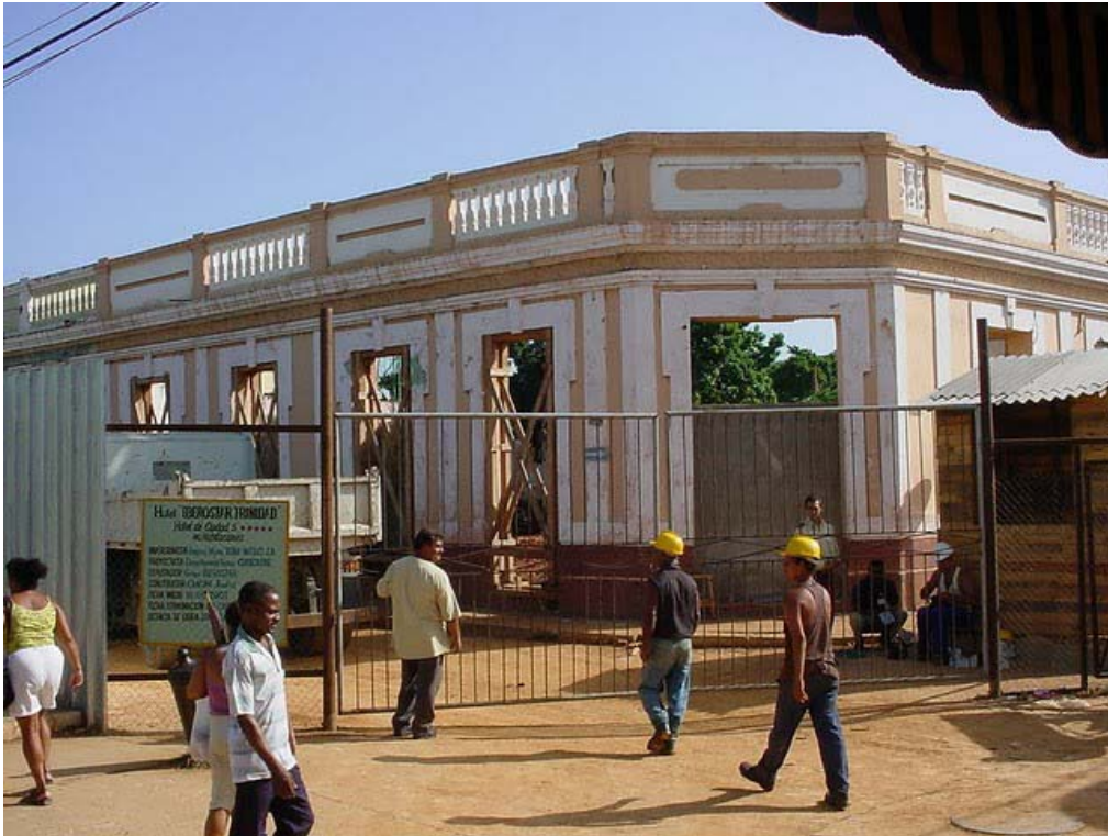
Figure 6.5 Hotel Iberostar construction. Photo by Carlos Sentmanat, used with permission from the photographer.
