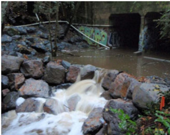
Figure 25. Water flowing through gaps in a boulder weir (Questa Engineering Corp 2009).
