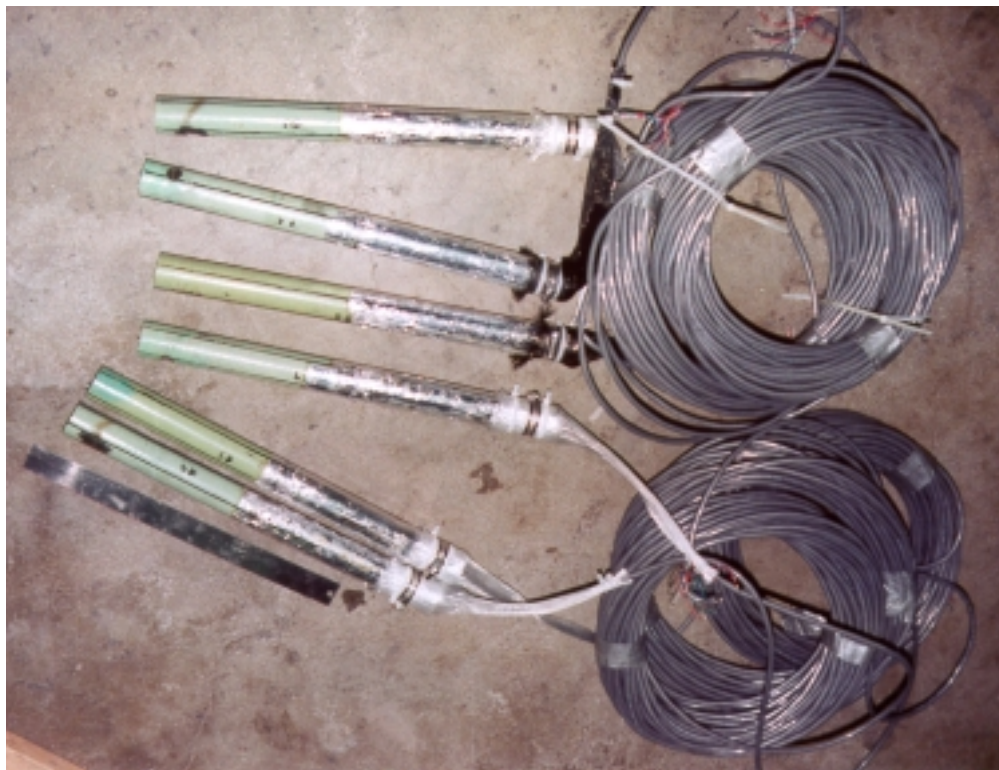
Figure 6.25. Individual Instrumented Dowel Bars Prior to being Welded to Dowel Bar Cage.
