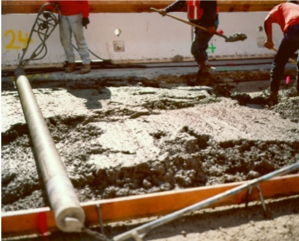
Figure 8.2. Unworkable Mix on South Tangent.
