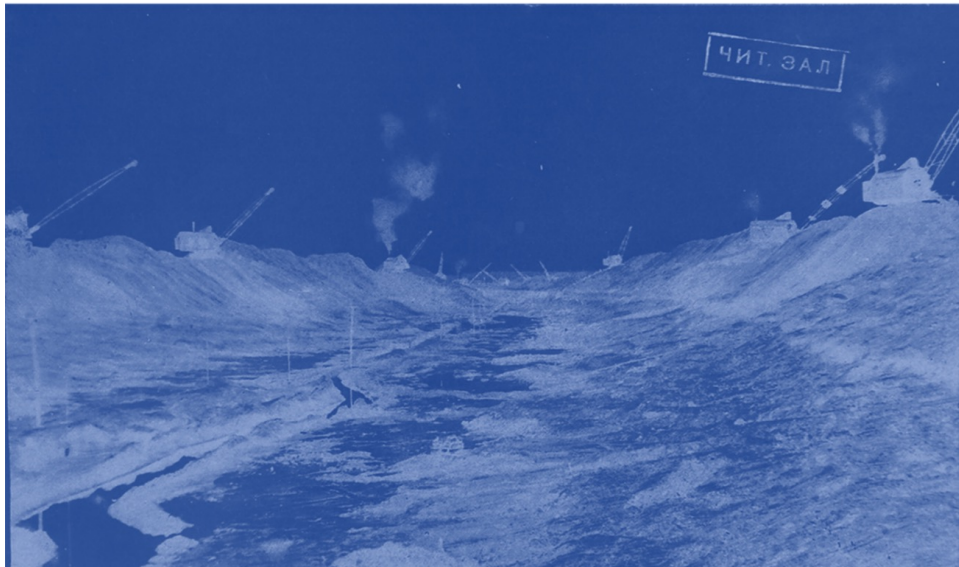
Figure 3. The trapezoid waterway bottom of the canal, 1936. Original image courtesy of Тypo-lytographia imeny Vorovskogo (Vorovskoy Printing House). Image edited by the author.
