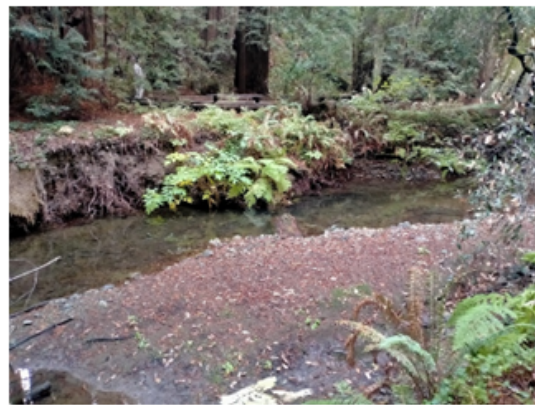
Fig. A9.3: Deep pool and bank erosion
