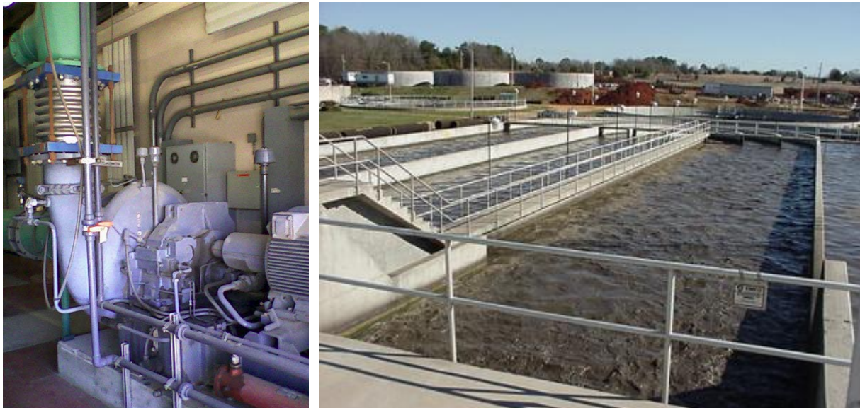
Figure 6: Blower (left) and an aeration basin (right).
