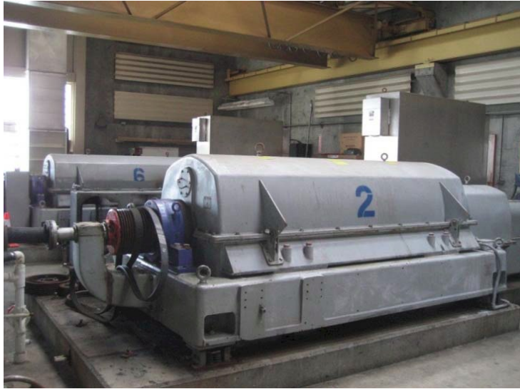
Figure 9: Example centrifuges used for sludge dewatering.
