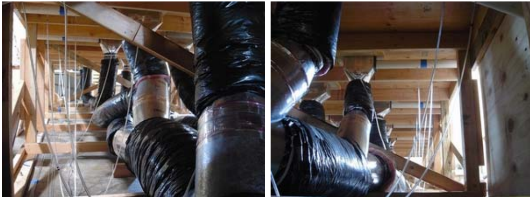
Figure 3. Ducts in the crawlspace below the test chamber.
