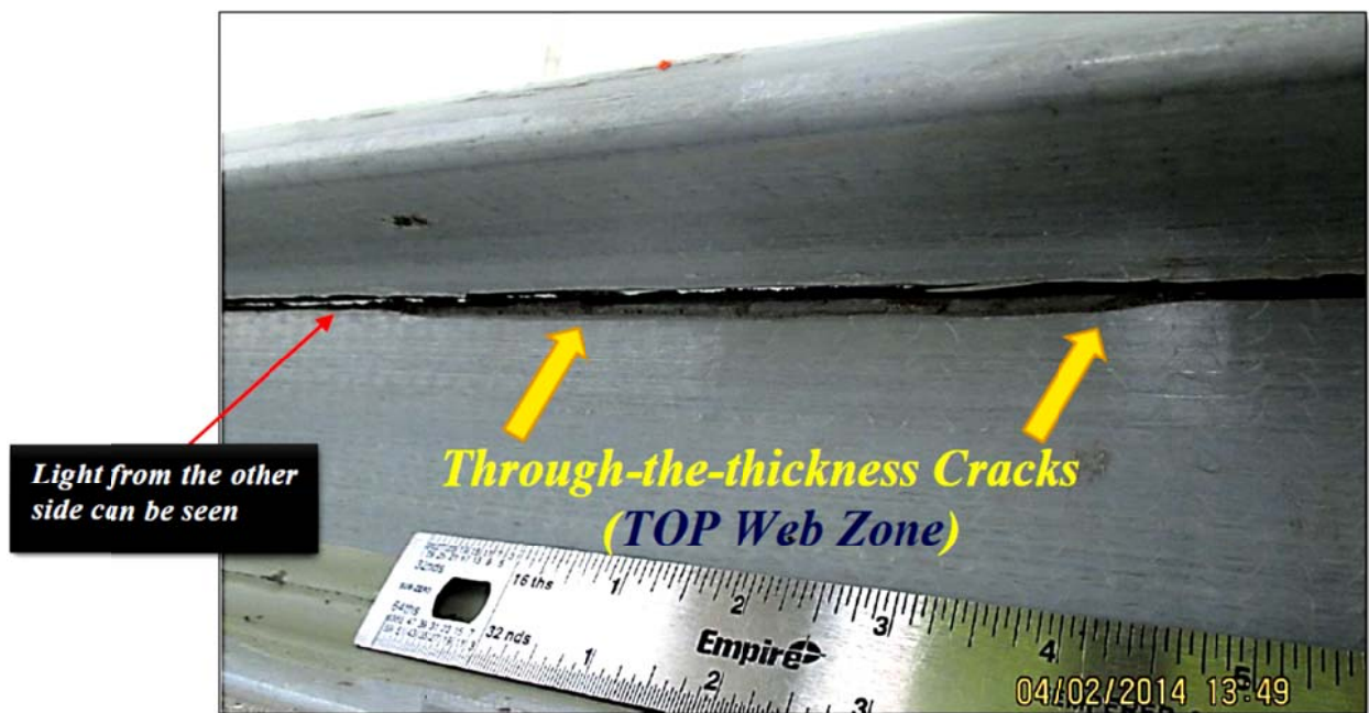
Figure (2): Web/Flange Failure of a Pultruded Composites Bridge Deck in USA
