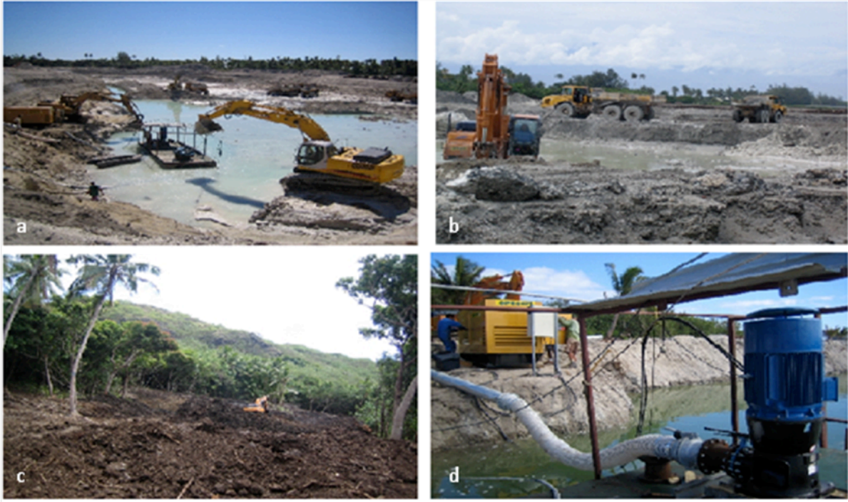
Fig. A2. Preparing the landscape for the golf course. Dredging and filling in of the lake (a) and (b), clearing of hillside (c), and pumping of lake (d). 2005-2006. Source: http://www.mooreagolf-resort.com .
