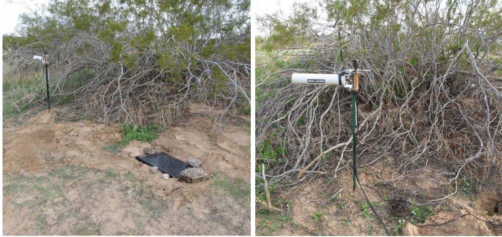
Figure 5.2: Photo of B003 and B004 unit installations at El Centro test site
