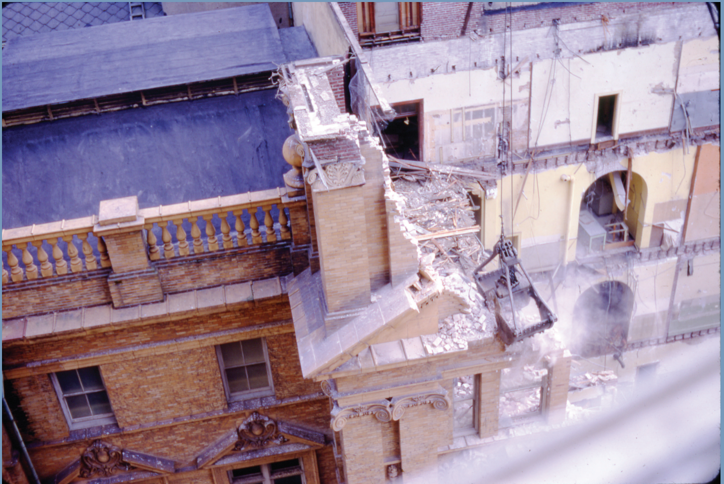
Demolition of old Medical School Building, 1967 with wrecking crane. From Robert L. Day Digital Image Collection, UCSF Archives and Special Collections.
