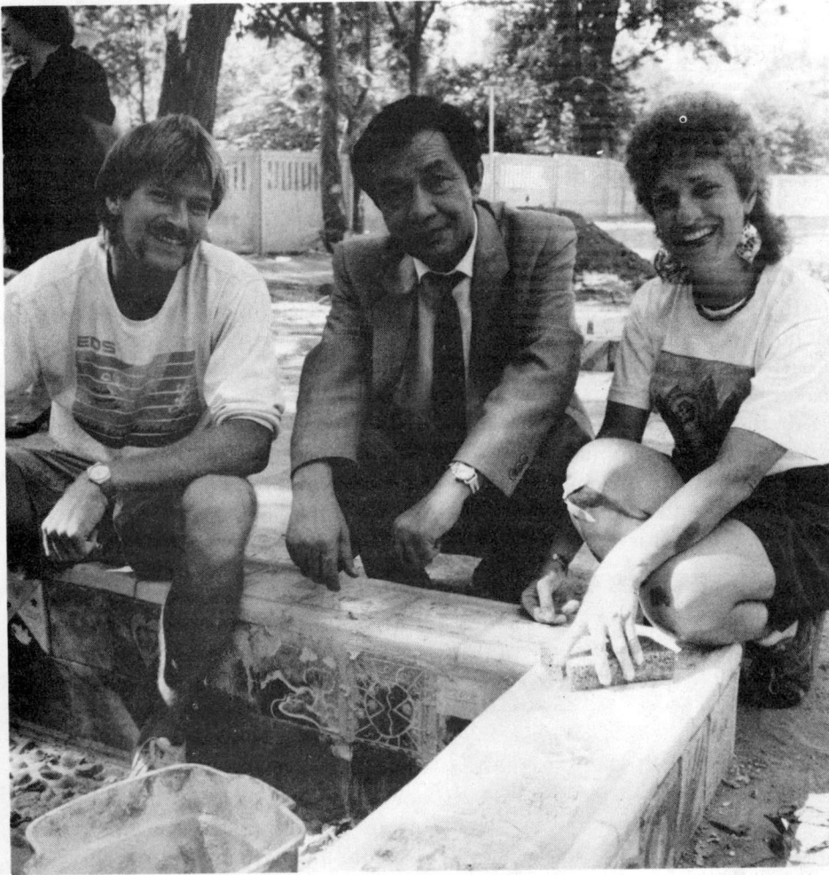
Tashkent Mayor Shukurulla Mirsayidov flanks Peace Park volunteers Dane Spencer and Mary Lynn Myer. Dane and Mary Lynn are taking a break from grouting tiles, an activity which took hundreds of hours.
