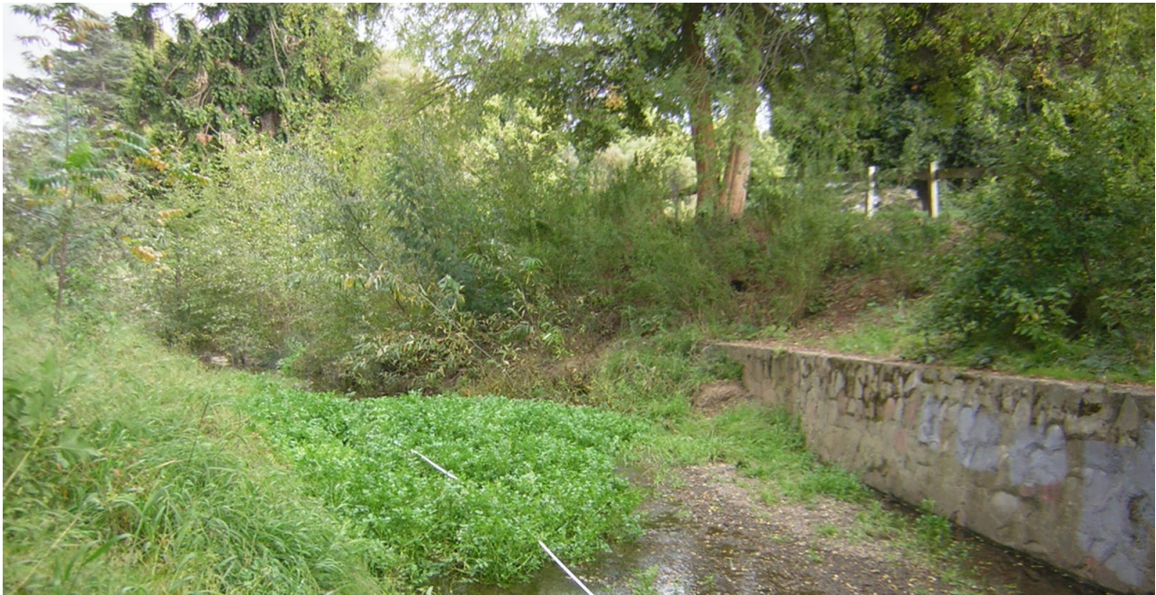
Photo 10. Looking toward the location of cross section III-III', which crossed the creek at the far end of the concrete retaining wall (along the right-hand side of the picture). Vegetation can be seen growing both on top of and at the base of the concrete retaining wall.
