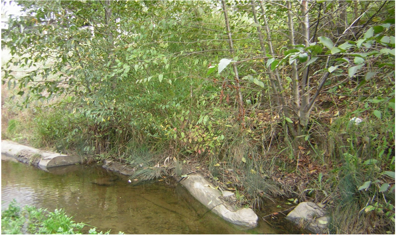
Photo 9. The installed log revetments have shifted and “floated” downstream as a result of inadequate restraint. Additionally, these logs do not provide significant scour protection during high flow events.
