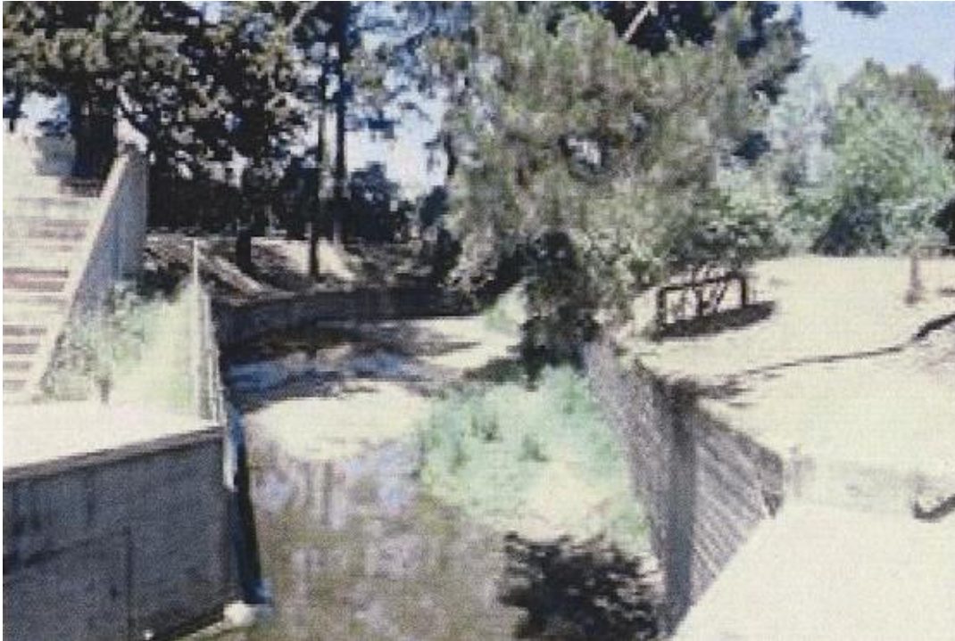
Photo 1. This pre-construction photo from Kupers (2001) shows the eastern stretch of the project reach, specifically the masonry and concrete channel walls that were targeted for removal. The view is upstream from the amphitheatre.
