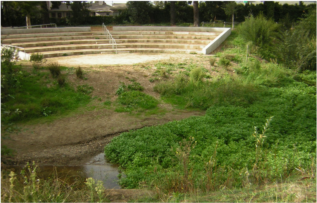
Photo 7. Reconstruction of the amphitheatre was one of the major components of the project. The amphitheatre, which formerly covered the creek with its stage, now transitions naturally into it, while providing a small floodplain for the creek.
