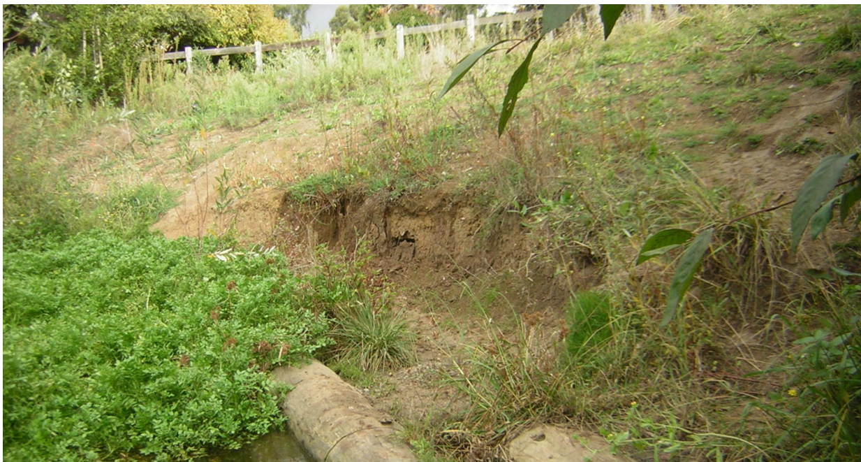
Photo 8. Significant scour is evident as a result of oversteepened creek bank slopes. The log revetments installed to mitigate bank erosion have shifted and moved during high flow creek events. In addition, these log revetments do not provide scour protection during high flow events.
