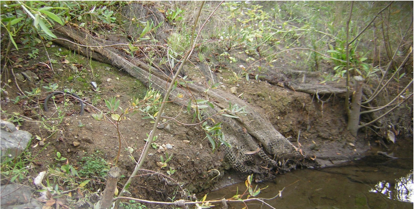
Photo 5. Erosion is evident immediately under the steel-framed pedestrian bridge as a result of the over-steepened creek bank in the vicinity of cross section B-B'. Active erosion is occurring behind the willow stakes.
