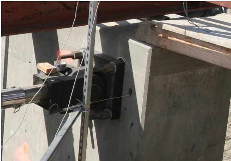
Figure 3.5. Photograph of horizontal LVDT attached between a metal bar extension and the test specimen
