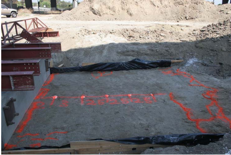
Figure 6.4. Photograph showing surface cracks across the backfill
