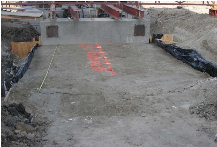
Figure 6.2. Photograph of second crack opening at 17 feet from wall face
