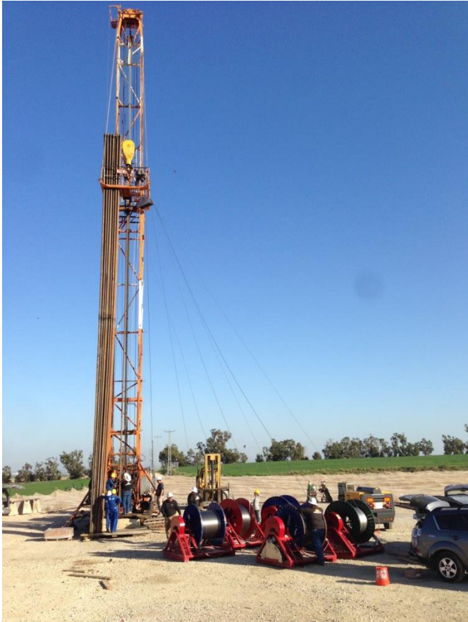
Fig. 8.4.3 Workover operation in progress at H18a showing rig with double stands of tubing and pneumatic spooling units used to tension control lines as they are fastened to the tubing.
