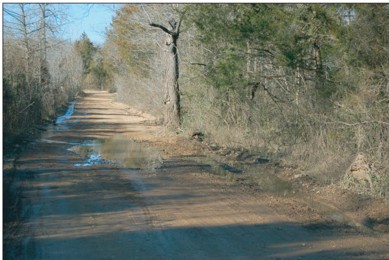
Figure 7. A location where a cross drain is needed to reduce sediment production.
