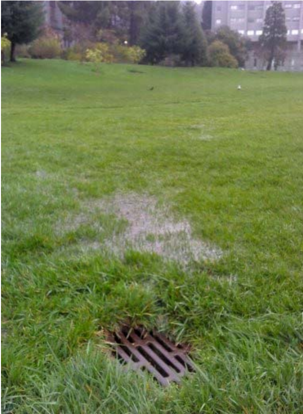
Figure 3: Runoff during a storm
