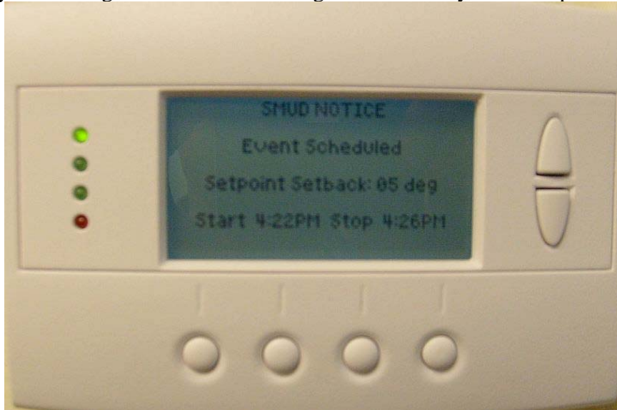
Figure 66. Programmable Communicating Thermostat Displaying Temperature Change Notice
