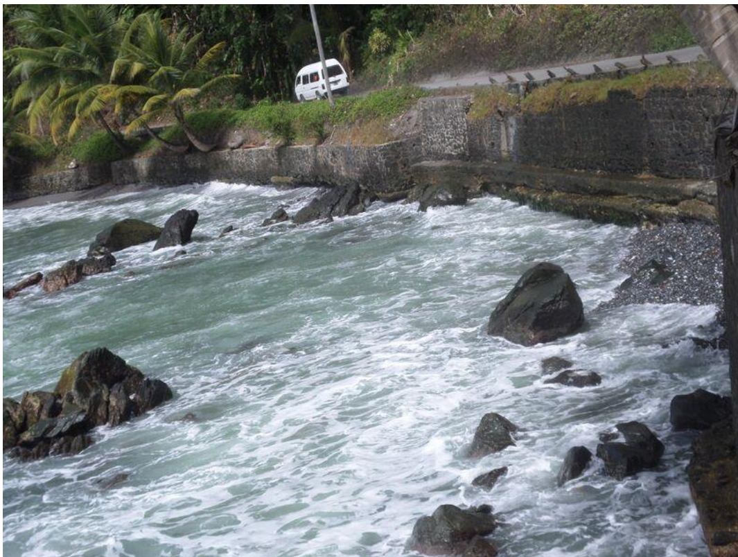
Figure 14. Road reinforced by sea wall which is being undermined wave action
