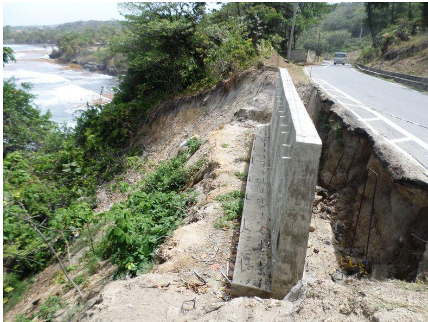
Figure 19. Damaged roadway and rehabilitative structure
