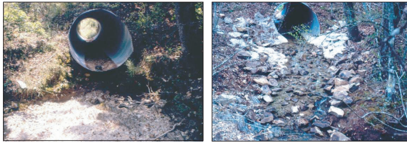
Figure 1. Rusted out pipe with drop. Figure 2. Grouted pipe and riprap ramp.
