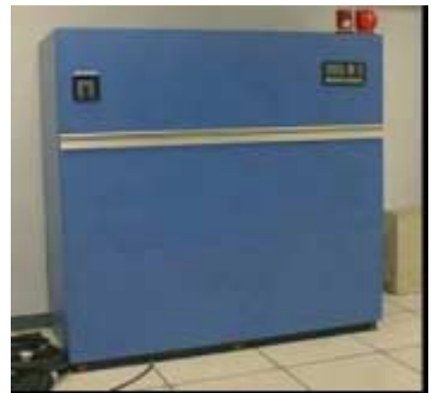
Figure 12 Typical CRAC unit
