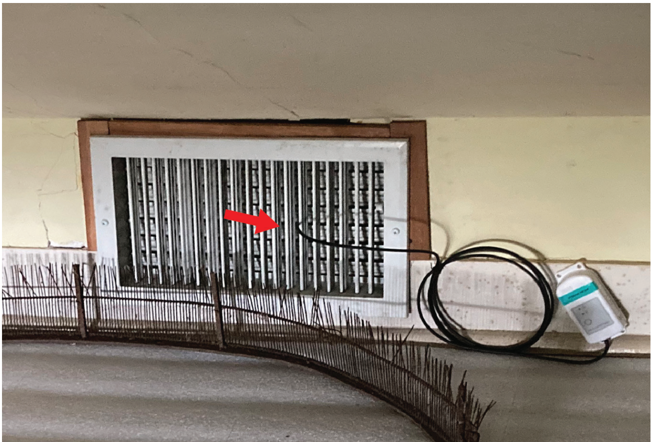
FIGURE 3 (above). Monitoring differential pressure between interior and exterior. FIGURE 4 (below). Monitoring temperature and relative humidity at supply register. DAVID BITTERMANN
