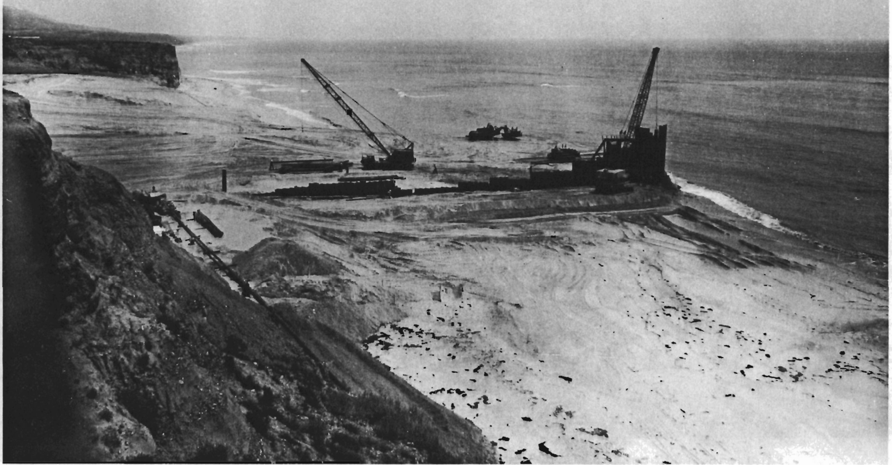
Figure 7. Photograph showing construction of north wall of Unit 1 laydown pad, taken on 4 June 1964 from Station "A".
