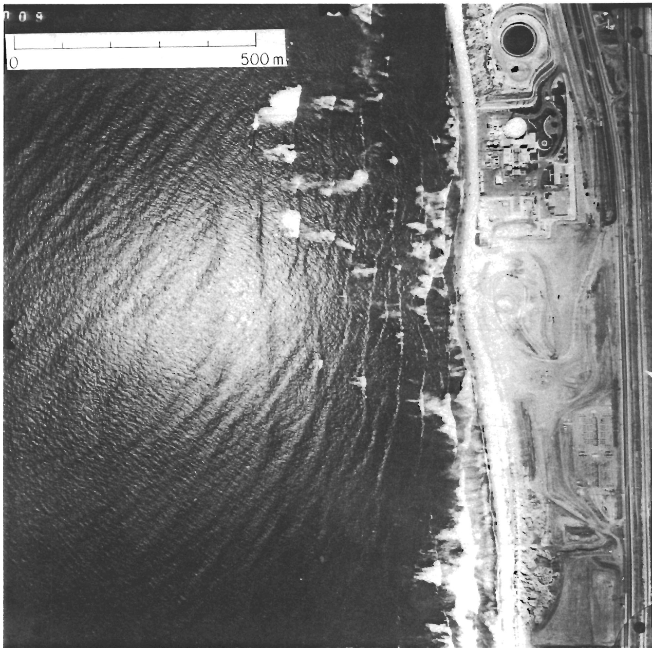
Figure 18. Aerial photograph of cliff excavation early in Units 2 and 3 construction phase, 17 May 1974.
