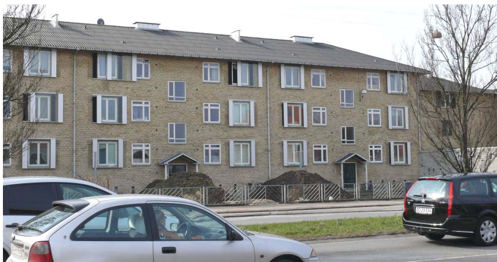
Figure 6.9. Noise reducing window constructed as a “noise shutter” that makes it possible to open the window. Placed in front of bedrooms and living rooms facing the highway (photo Allan Jensen, Rambøll).
