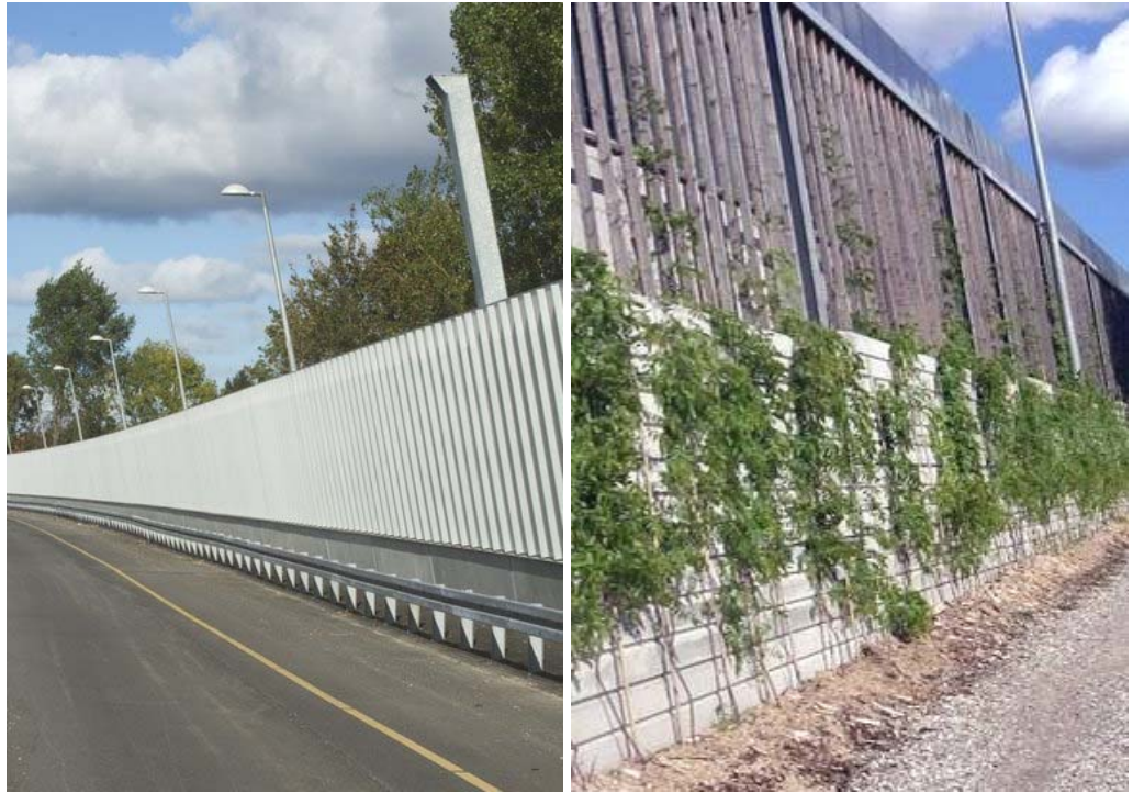
Figure 5.4. Close up of the noise barriers designed for the M3 project (roadside left and urban side right).
