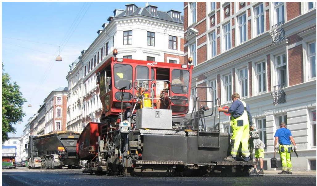
Figure 2.1. When road construction work is carried out in close proximity to residential areas, it is relevant to consider construction noise when planning and realizing such works.
