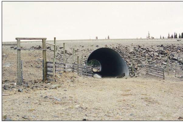
Figure 5. Wildlife underpass designed for deer on the Okanagan Connector (early 1990's).
