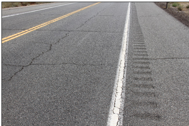
Figure 4.1: SBD-2: Transverse and longitudinal cracking.
