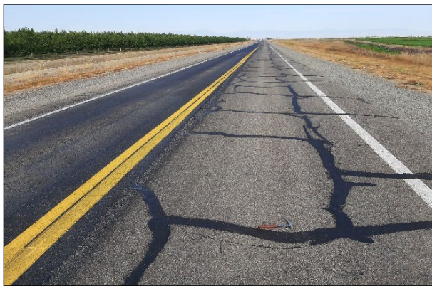
Figure 2.1: GLE-162: Alligator B cracking.
