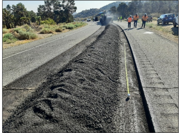
Figure 4.6: SBD-2: Spacing of transverse cracking.
