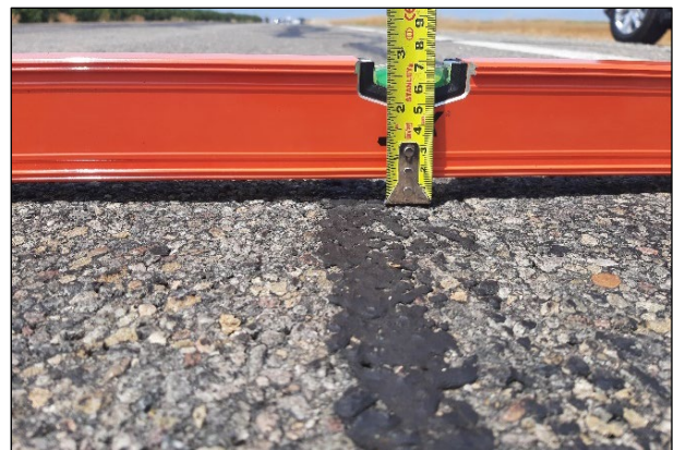
Figure 2.4: GLE-162: Wheelpath rutting.
