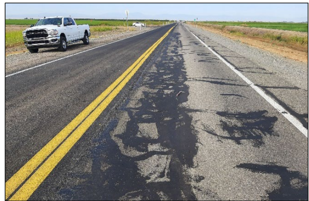
Figure 2.2: GLE-162: Alligator C cracking.
