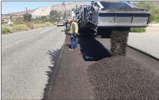
Figure 4.10: SBD-2: Emulsified asphalt spilling out of recycling chamber.
