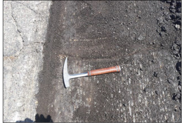
Figure 3.14: SB-135: Reflected transverse cracks in cut.
