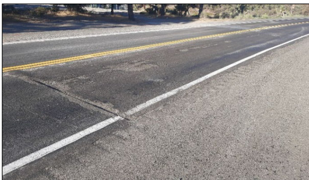
Figure 4.12: SBD-2: Raveling of PDR-EA layer constructed at end of day - 08/31/21.
