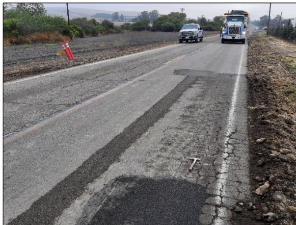
Figure 3.7: SB-135: Severe alligator cracking along the edge of the pavement.
