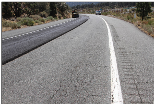
Figure 4.3: SBD-2: Alligator B cracking in the wheelpaths.
