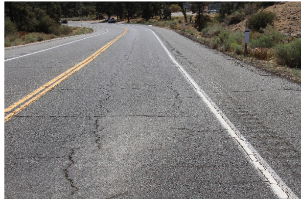
Figure 4.2: SBD-2: Block cracking.
