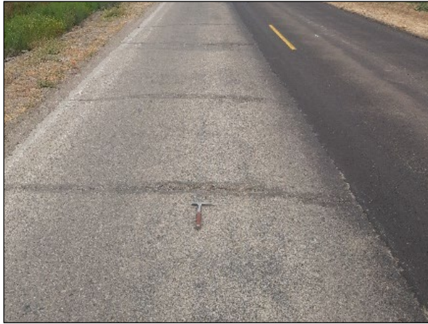
Figure 3.3: SB-135: Transverse cracking.
