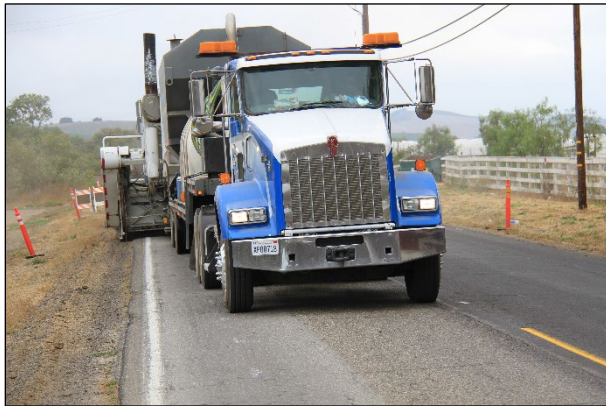
Figure 3.11: SB-135: Narrow lane showing center overlap and milling of shoulder material.
