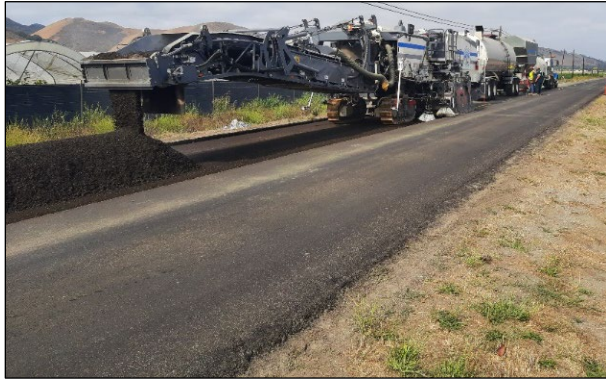
Figure 3.8: SB-135: Single-unit recycling train. (Water tanker and cement spreader, asphalt tanker, recycling unit).
