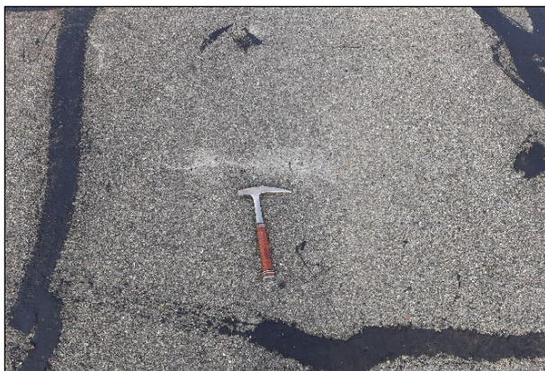
Figure 2.3: GLE-162: Pumping of fines through unsealed cracks.
