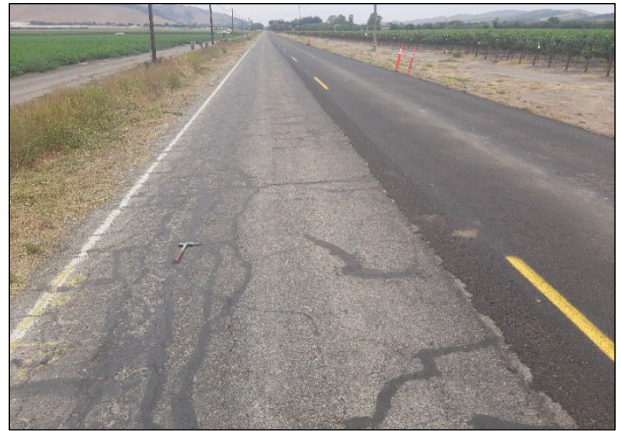
Figure 3.6: SB-135: Sealed Alligator B cracking.
