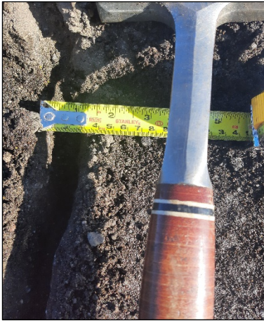
Figure 4.5: SBD-2: Width of reflective transverse shrinkage cracks in cut.
