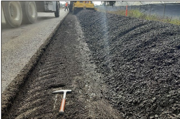
Figure 3.15: SB-135: Layer of fine material in the cut next to the windrow.
