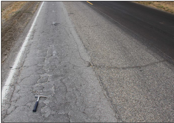
Figure 3.5: SB-135: Alligator B cracking.
