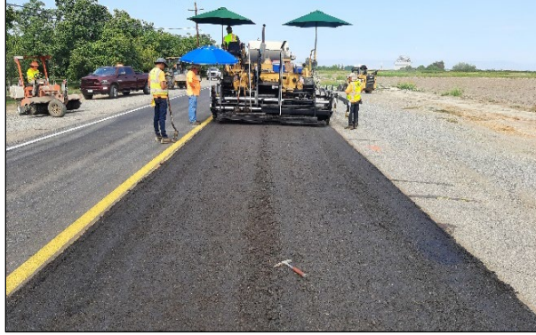
Figure 2.22: GLE-162: Segregation along centerline of lane behind paver.
