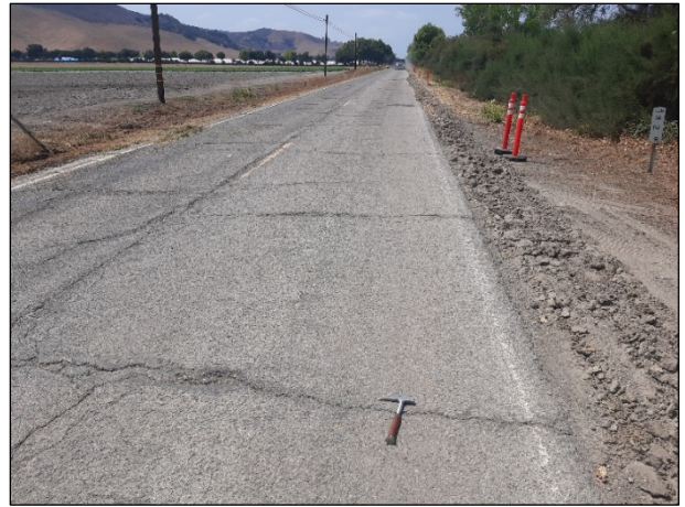
Figure 3.4: SB-135: Spalling on cracks.
