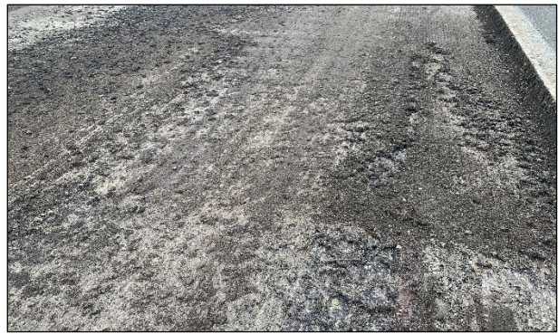
Figure 4.8: SBD-2: Remains of asphalt rubber chip seal SAMI at bottom of milling cut.
