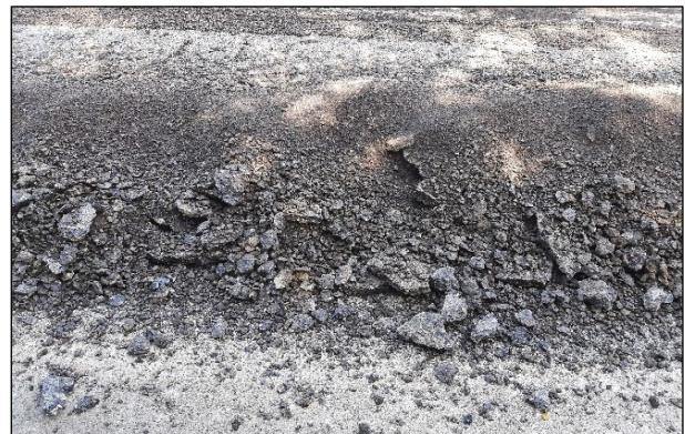
Figure 3.18: SB-135: Oversize RAP from milling loose blocks in fatigue cracked areas.
