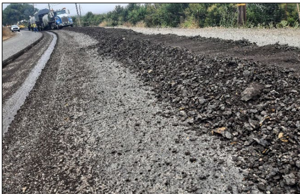
Figure 3.17: SB-135: Oversize RAP from incorrect pre-milling speed.
