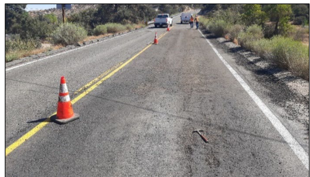
Figure 4.13: SBD-2: Raveling of PDR-EA layer constructed at end of day - 09/01/21.
