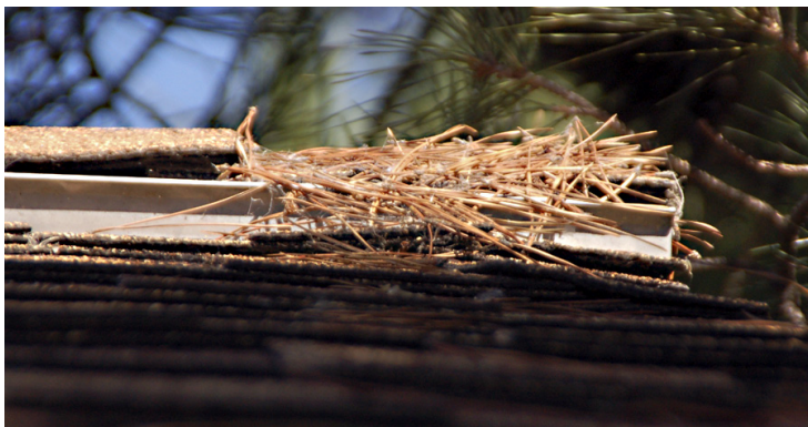
Figure 11. Accumulation of pine needles at the entrance to a ridge vent. Photo: Stephen L. Quarles.
