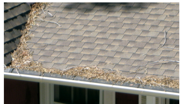
Figure 8. Debris accumulation behind a gutter cover device. The gutter is clear of debris, but the roof still should be cleared of debris. Photo: Stephen L. Quarles.
