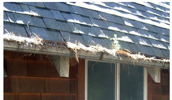
Figure 7. Note the heavy needle accumulation in this metal gutter. If ignited by embers, flames would impinge on the roof edge, potentially igniting the roof sheathing. Because of the open eave construction (i.e., exposed rafters), the fire would not immediately enter the attic or cathedral ceiling space. If ignited, the wood shingle siding and plywood skirting also shown in this photograph would threaten the home via a flame contact exposure to the single-pane window and the under-eave area. The ignited shingle siding could also burn into the stud cavity and into the living space of the home. Photo: Stephen L. Quarles.
