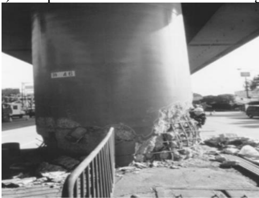
(c) Column shear failure
