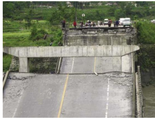
(b) Abutments fell
