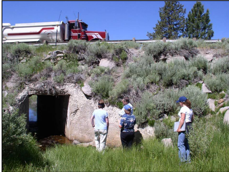
Figure 3. This site was chosen as the highest-priority location for an improved underpass suitable for all local species. Instead of replacing this box culvert, Caltrans engineers suggested installing an additional underpass 5 meters to the right of this view because of reduced installation costs. Image by Michael DeLasaux.
