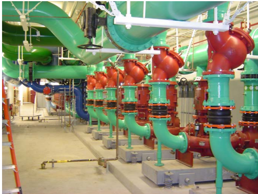
Figure 3. Primary condenser water pumps.
