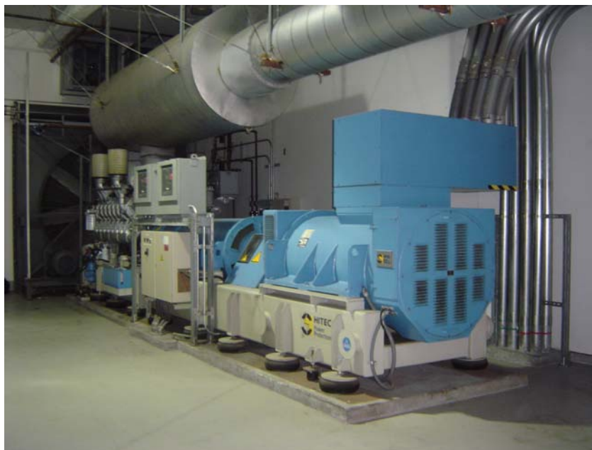
Figure 1. Typical HITEC Diesel UPS/Backup Generator.
