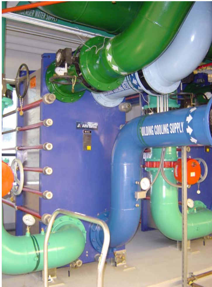
Figure 4. Heat Exchanger for condenser water.
