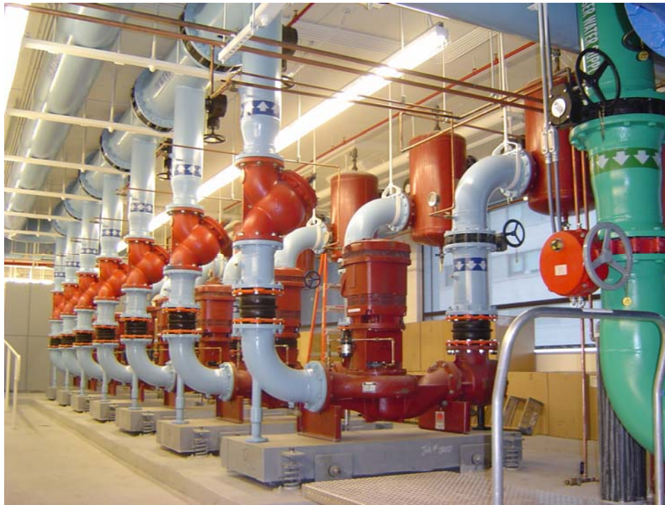
Figure 5. Secondary condenser water pumps.
