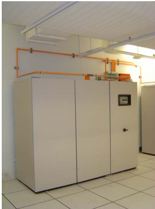
Figure 6. Sample CRAC Unit
