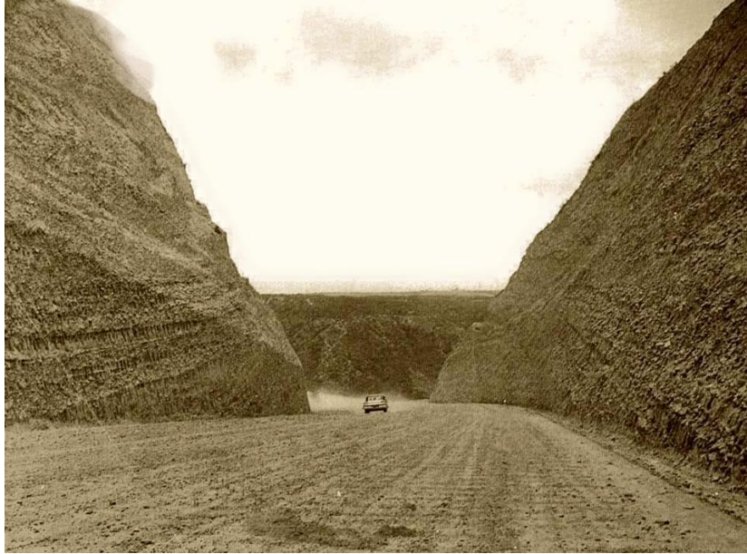
Figure 1-04 shows the cut of the mesa. The picture was taken within the cut area, looking back to the east (Por las calles y colonias de Tijuana, 2002).
