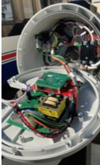
Figure 18: Aerovironment Level 2 Smart PEV Charging Device
