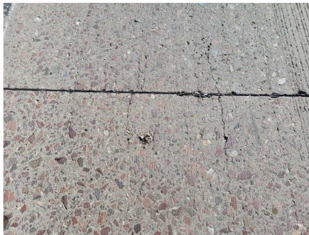
Figure 3.7: Low severity longitudinal cracking at wheelpath, I-40-Ludlow.
