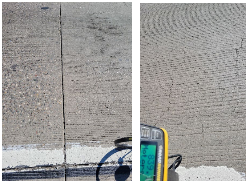
Figure 3.5: Map cracking (left) and transverse cracking (right), I-15-Victorville.
