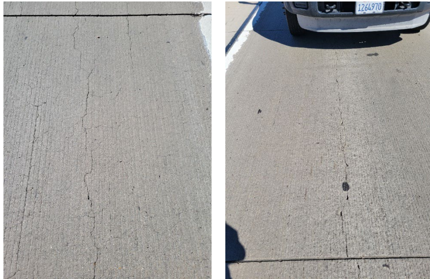
Figure 3.4: Low severity longitudinal cracks, I-15-Victorville.
