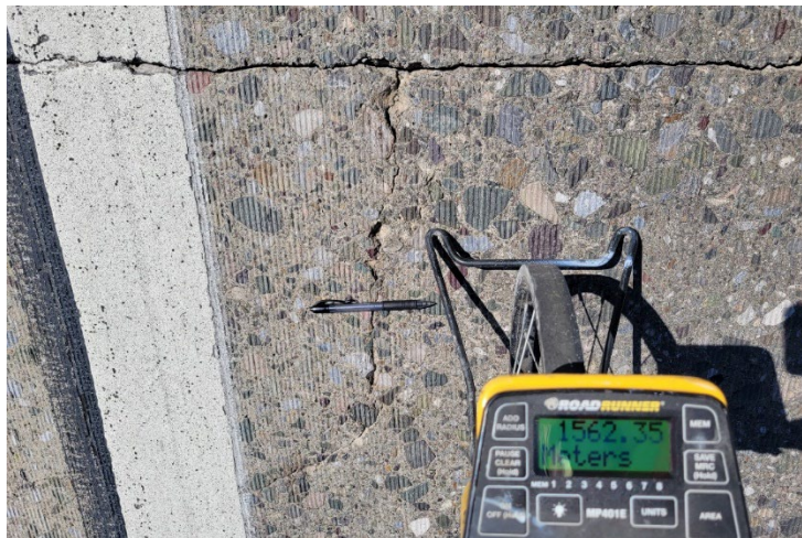
Figure 3.2: Corner crack, I-15-Baker.
