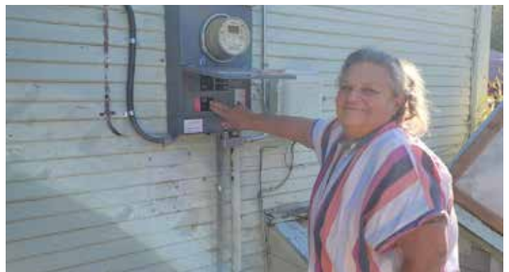
Patricia Barrett flips the switch to turn on new GRID Alternatives solar panels on her home. Photo credit: Patricia Barrett
