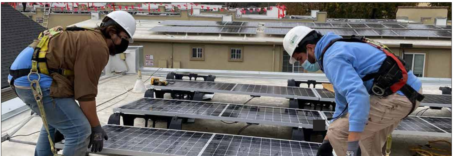
Solar installers from GRID Alternatives laying down PV modules at Casa de Oasis. Photo credit: GRID Alternatives
