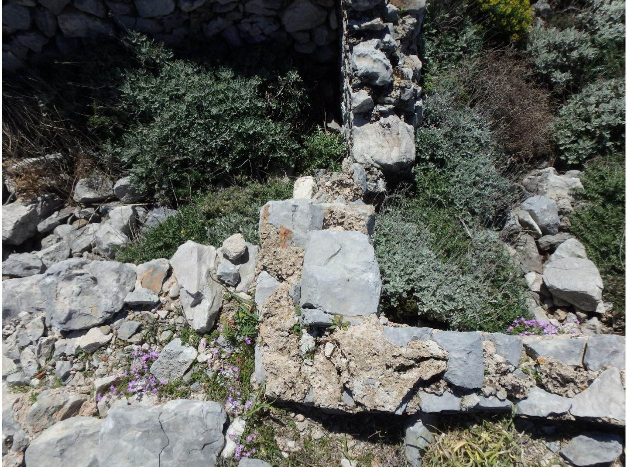
Figure 120: Detail of multiple building phases in cistern complex at center of Tigani. (Photo: M. Pawlowski)
