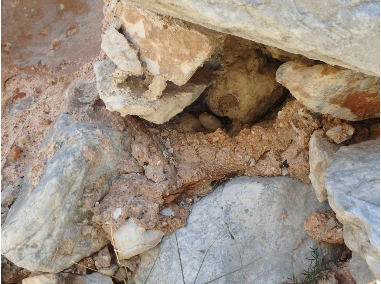
Figure 126: Chunky pink mortar in lower wall of cistern near House 5 at Tigani. (Photo: M. Pawlowski)
