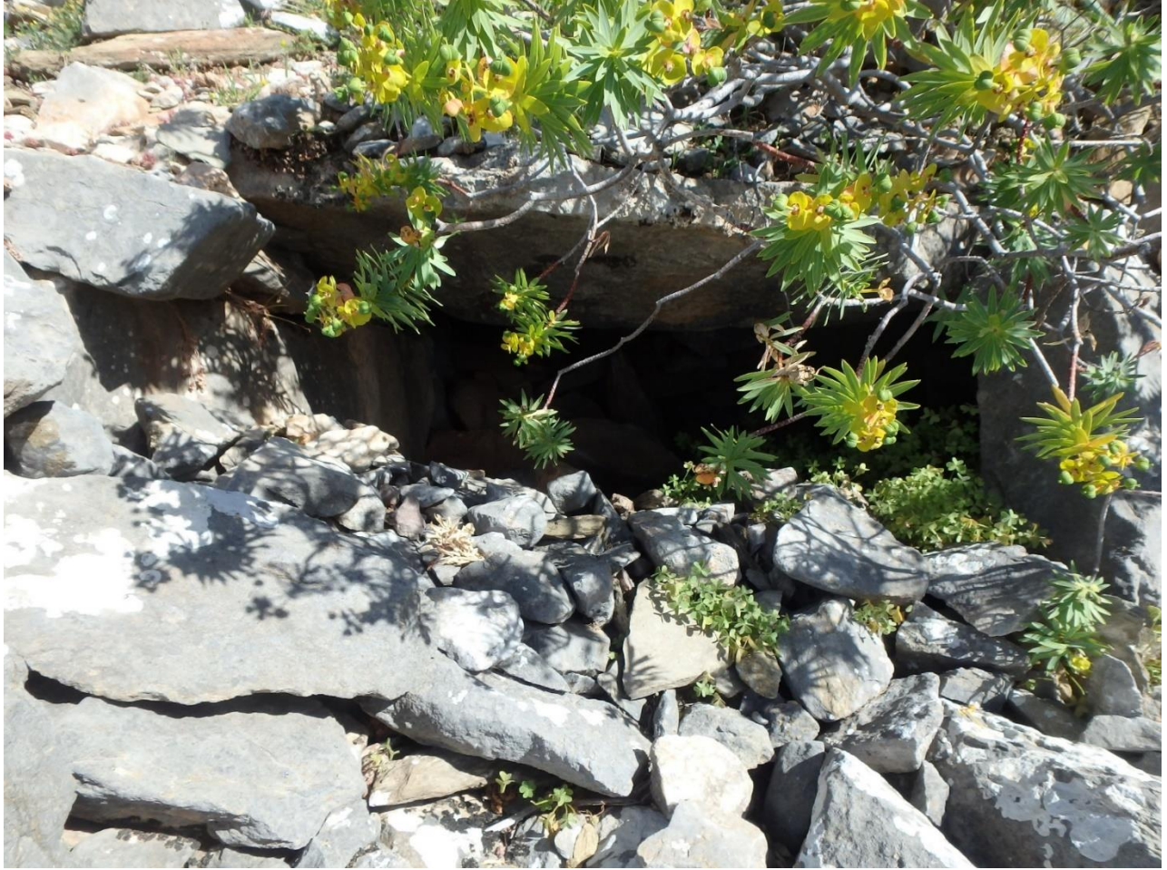
Figure 226: Preserved ceiling to addition of House 26 from the south. (Photo: M. Pawlowski)
