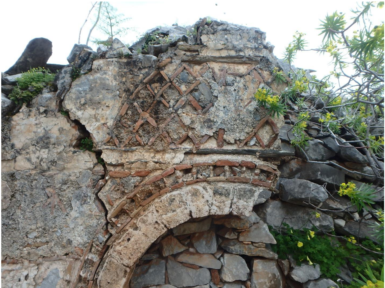
Figure 50: Brickwork on original western facade of Hagia Kyriaki, Marathos. (Photo: M. Pawlowski)
