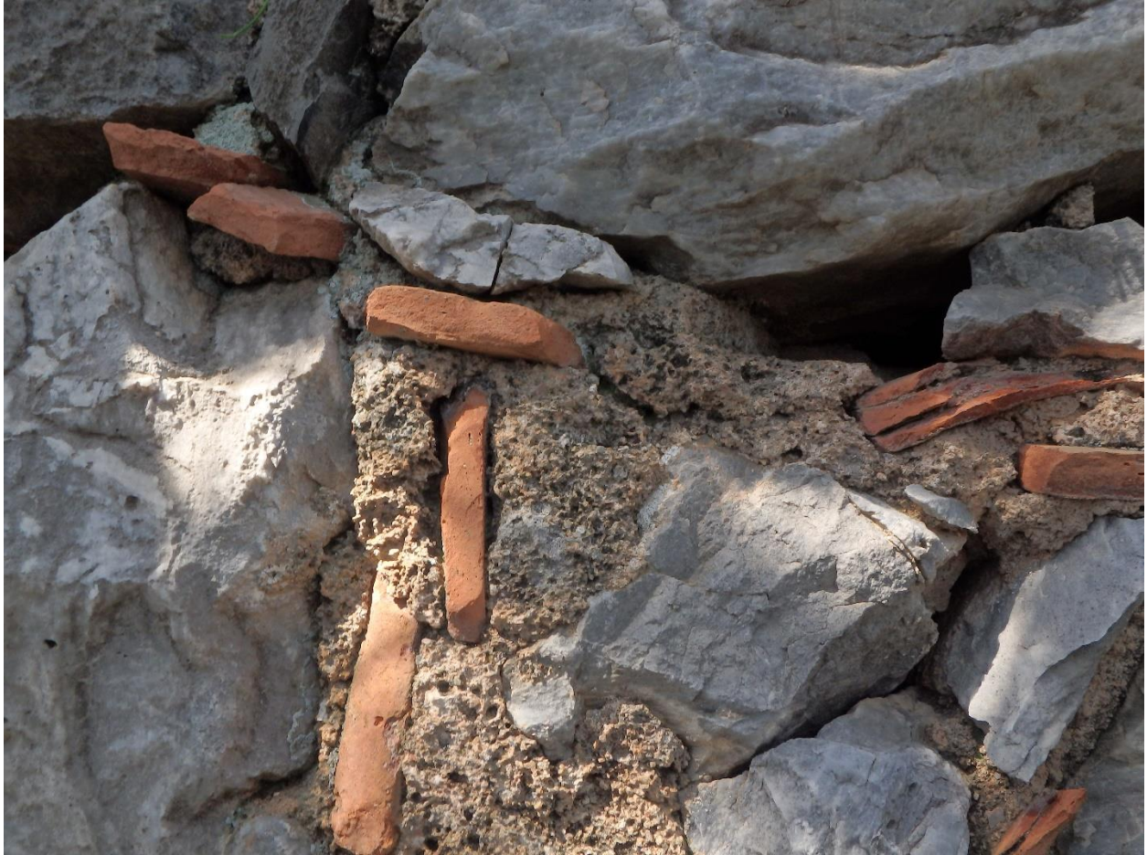
Figure 63: Detail of brick and mortar from north wall of Church C, Marathos. (Photo: M. Pawlowski)
