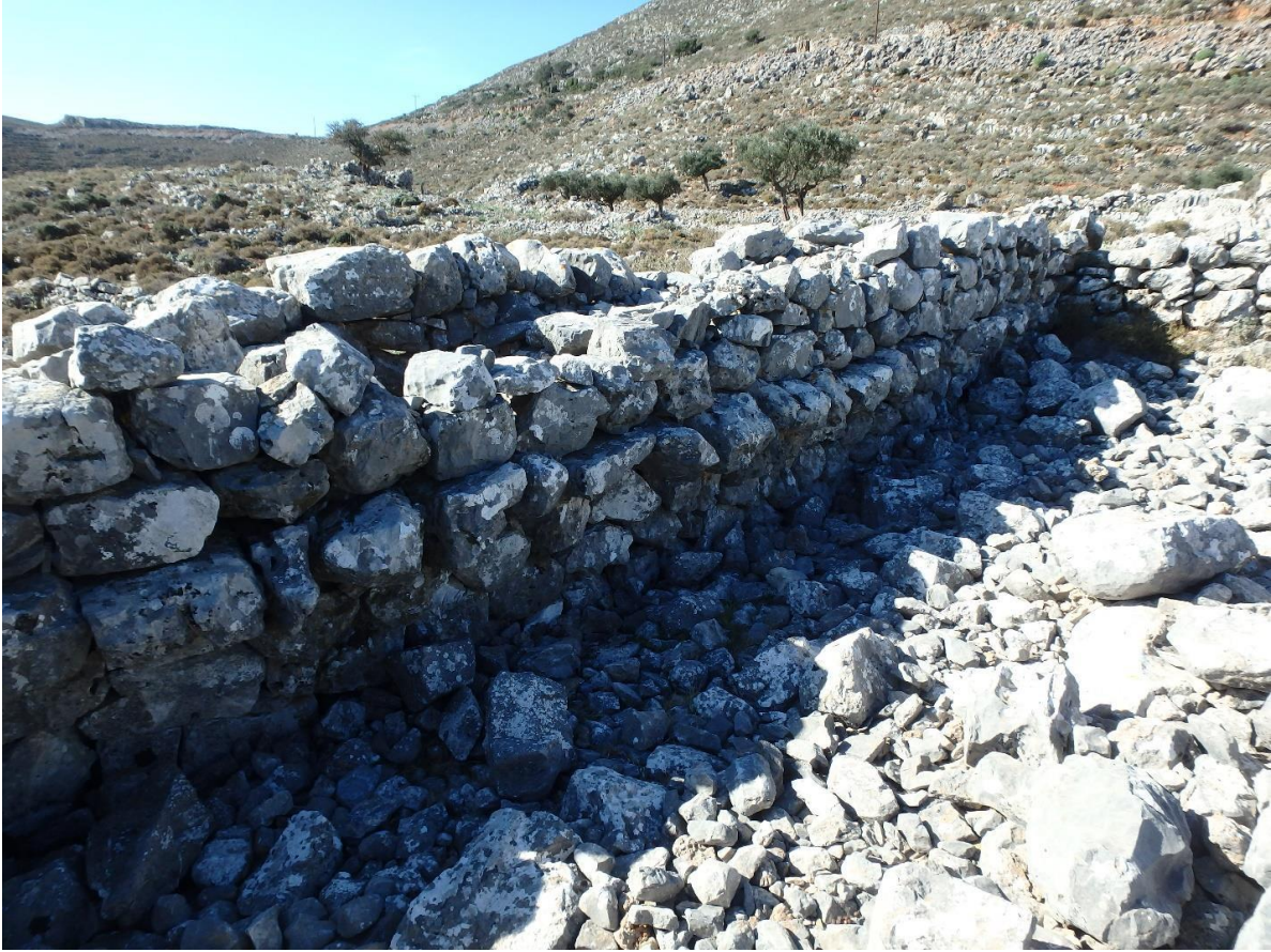
Figure 28: View of House 6, Sarania from the north with joist hangers visible on south wall. (Photo: M. Pawlowski)
