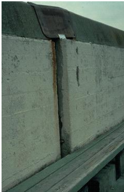
Figure 3-7. Displacement of the U.C. Berkeley Memorial Stadium wall as a result of the movement of the Hayward Fault
