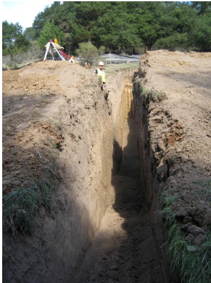
Figure 3-53. View to the east of trench NUMO TR1 before hydraulic shoring was placed.
