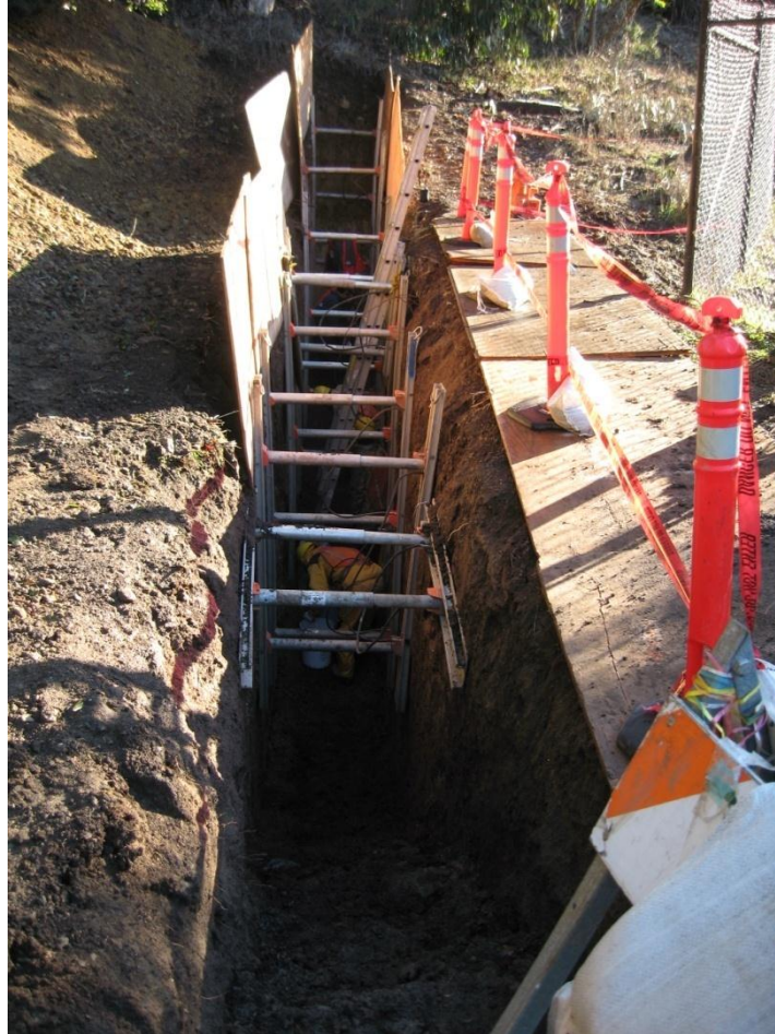
Figure 3-55. View to the east of trench NUMO TR2 near the north gate to the Fire trail.
