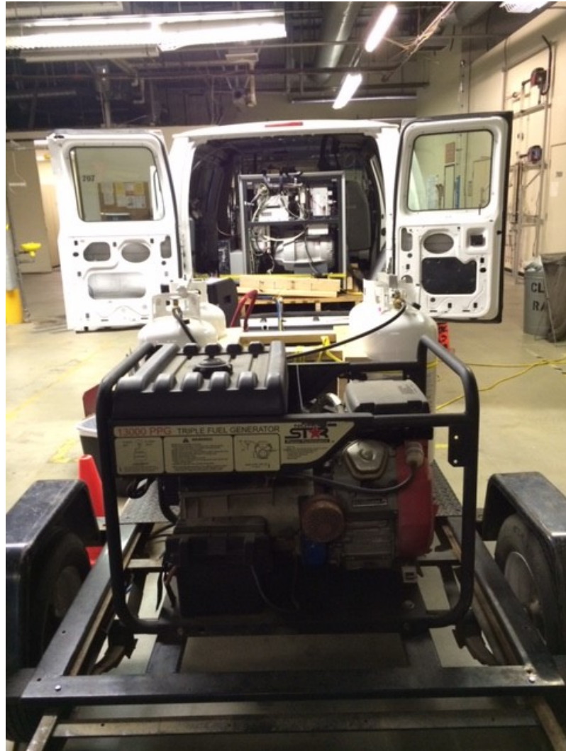
Figure 2.12: System Power for Mobile Laboratory I
