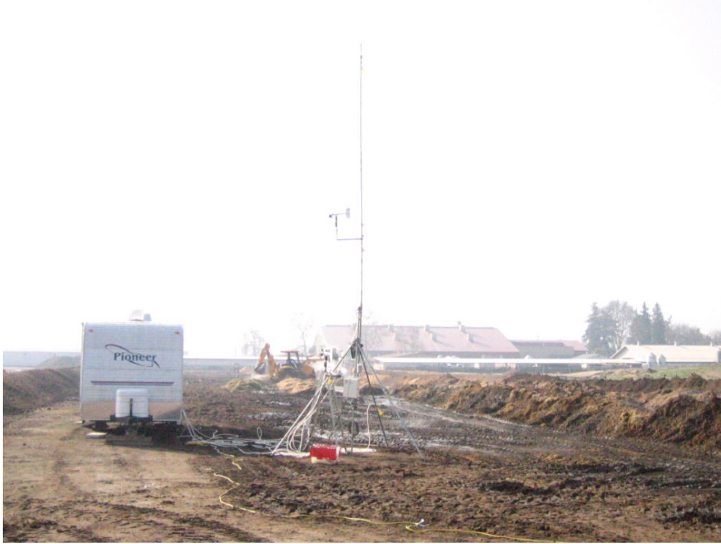
Figure 46: Instrumentation Trailer (left) with Sensor Tower (2/9/08) over the disturbed compost pile, notice backhoe in rear of figure
