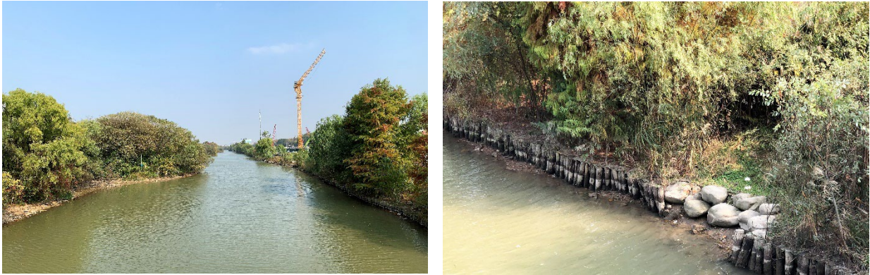
Figure 8: River channel at transect S2: aerial view (left) and bank protection measures (right)
