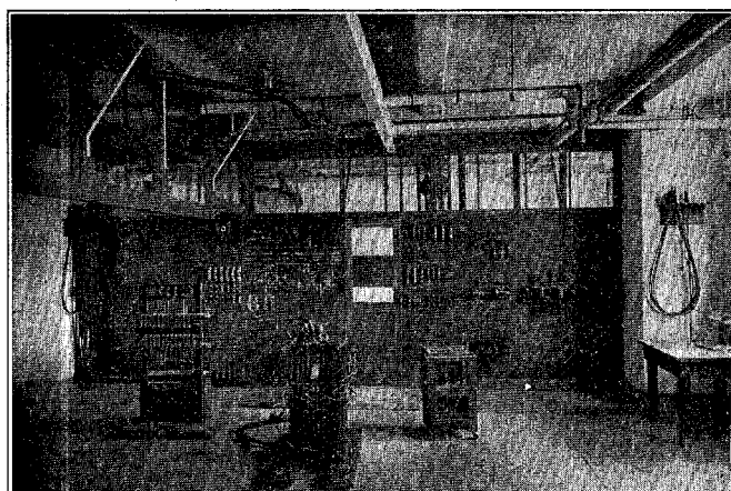
FIG. 9—ELECTRIC FURNACE LABORATORY, ROOM 19. FEEDER PANEL (UNFINISHED) BEHIND WHICH ARE THE MOTOR GENERATORS AND OIL SWITCHES
