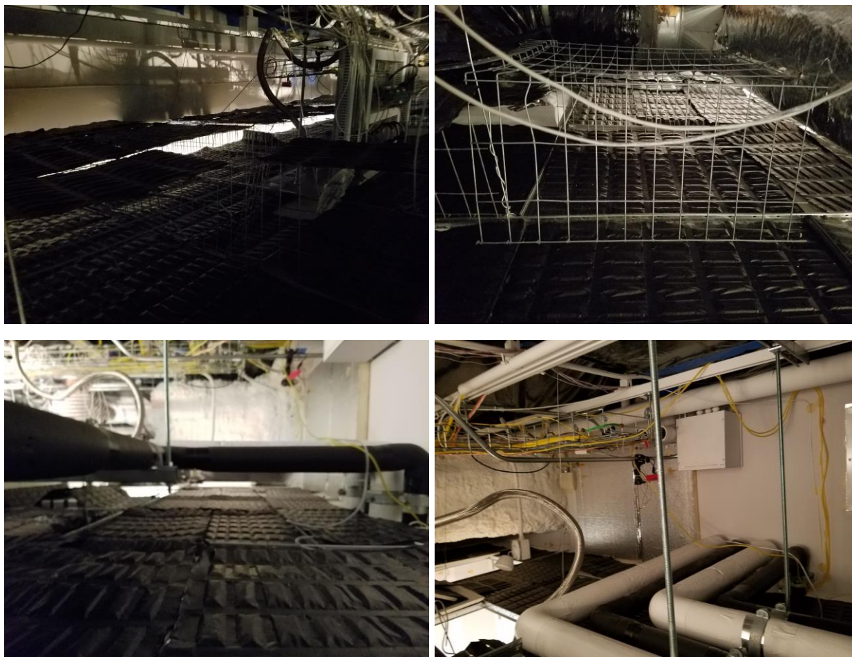
FIGURE 4 : ROUND 2 PCM INSTALLED IN FLEXLAB PLENUM (COURTESY OF ROB MORTON)
