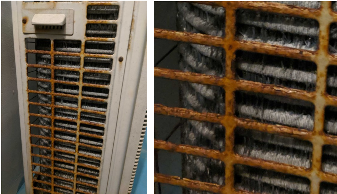
Figure 2: Air conditioning unit showing signs of corrosion (left). The expanded picture of the coil shows loss of fins and accumulation of corrosion products that affect system efficiency (right).
